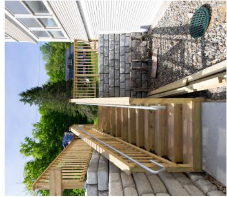
Stairs to lower parking built as part of rehab at Newport's Lakeview Housing
